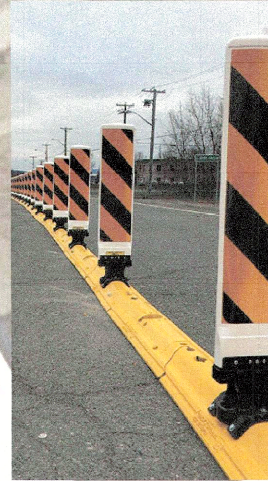
PHASE 1 - INSTALLATION OF QWICK KURBS AT MIDDLE SCHOOL NORTH SIDE CROSSING ON US-12. PHASE 2 WOULD INSTALL PERMANENT CURB WITH MDOT APPROVAL AFTER TRIAL PERIOD.
